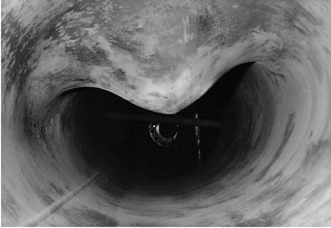
10.2 Dent (probable cause: construction or agricultural equipment).
