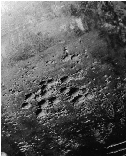
10.3 Pitting corrosion (external).
