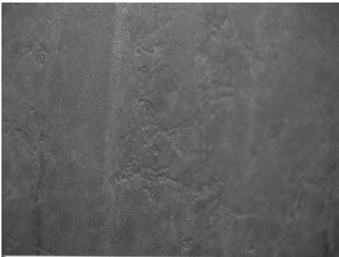
1.7 Uniform or general corrosion on pipe surface.
