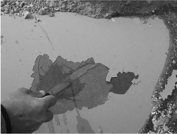
1.14 Fusion-bonded epoxy coating systems are known to be ‘non-shielding’ to CP current if disbondment or blistering occurs, therefore it is rare to find external corrosion or SCC on FBE coated pipelines with adequate CP. Photo shows poor adhesion and water under blisters, but no corrosion and a pH of 12.
