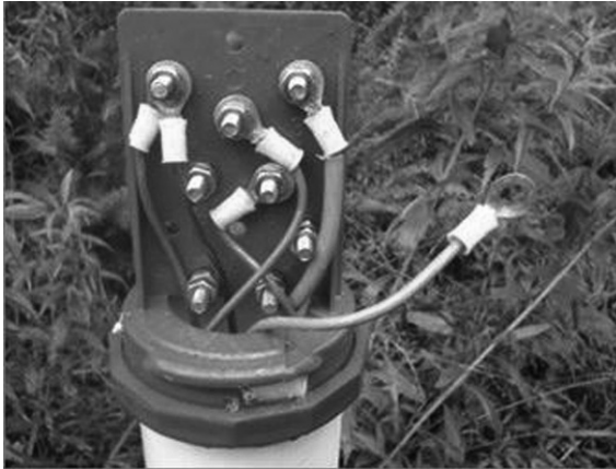
8.10 Multiple wire pipeline test station.
