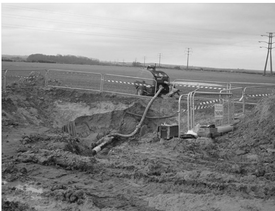
2.1 Pipelines in the vicinity of high voltage electric power lines.
